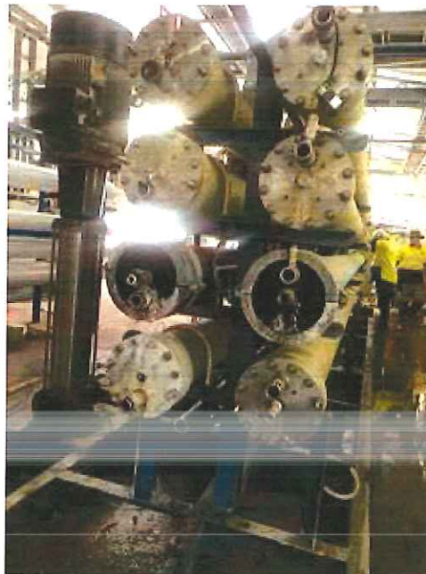
Old reverse osmosis system
