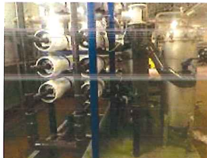
New reverse osmosis system
