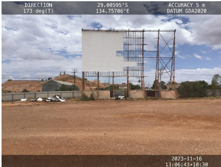
2. Coober Pedy Gym/Sport Centre – part of the veranda was torn from the building.
